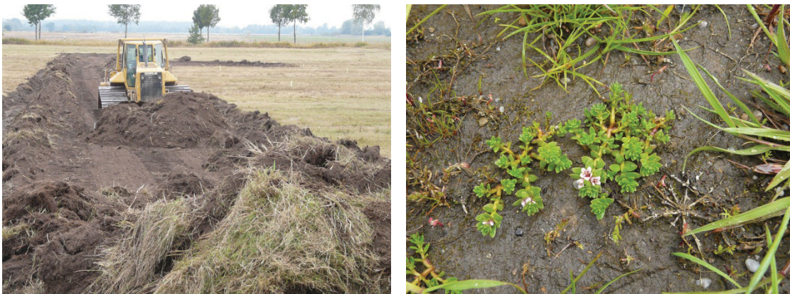
Figure 12 and : Removal of the strongly rooted and nutrient-rich top soil with heavy machinery (left); afterwards: typical halophytes like Sea Milkweed ( Glaux maritima ) (right) spread on the area. Source: Dieter Leupold
